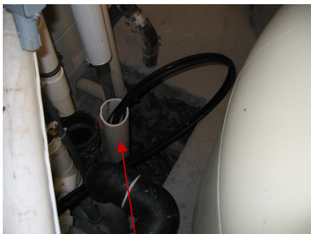
Conduit into mechanical room
